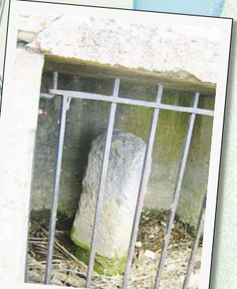
The eroded stub of the south cornerstone sits inside the seawall under Jones Point Lighthouse , which once guided ships along the Potomac.
